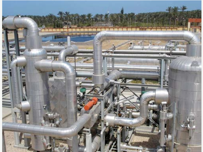
Dana Gas Egypt's El Wastani gas-processing facilities in the Nile Delta. www.danagas.com
