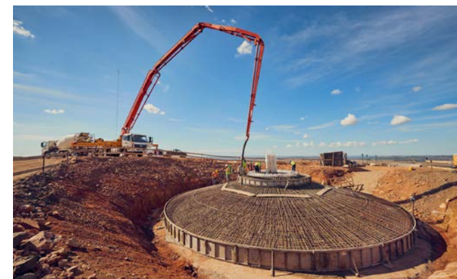
Ingener worked on the 50 MW Parque Eólico Melowind project
